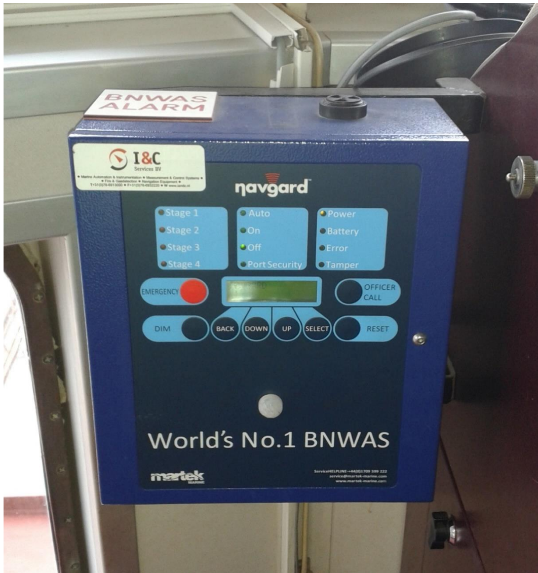
Figure 16: BNWAS control panel, installed at waist level on the port side directly adjacent to the bridge control console (see Figure 17). The status and operating display is located in the centre, with three groups of four status lights positioned above it. As the device shown is switched off, the green 'Off' status light is illuminated. Below that, there are eight keys to the left and right of the display. The reset key is bottom right, while the red emergency call key is top left. The white 'key' in the centre above the text 'World's No. 1 BNWAS' is the lens of the built-in infrared motion sensor.
