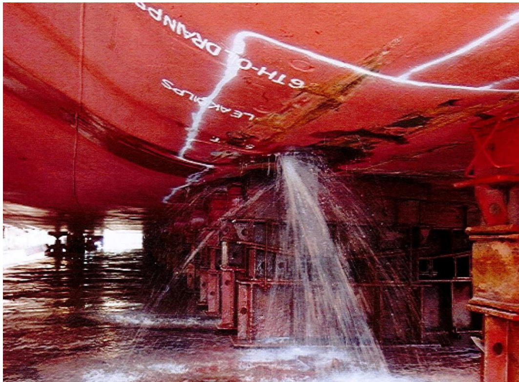
Figure 11: SABINA in dry dock in Tallinn. View from aft towards the bow. Breaches, dents and scratches in the areas of the port-side double bottom water ballast tank and pipe tunnel, as well as dents and scratches in the areas of the port-side double bottom water ballast tank, pipe tunnel, leak oil tank (marked 'LEAK OIL PS') and thermal oil drain tank (marked 'OIL DRAIN PS'). The water that had entered SABINA's double bottom pours out of the breaches in the double bottom and onto the drained dry dock.
