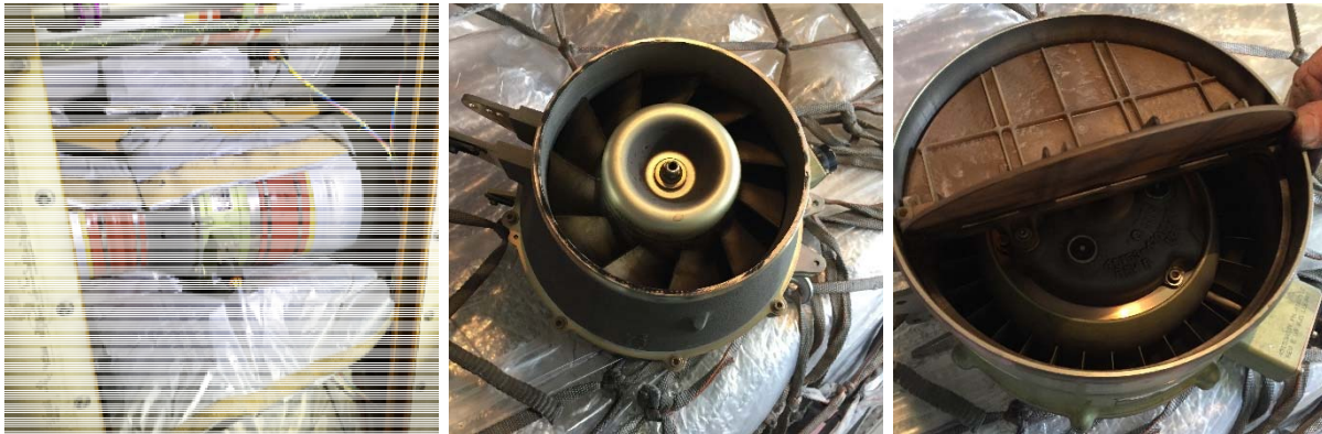
Figure 3: Image on the left: cooling fan on the left sidewall of the forward cargo compartment. Image in the middle and on the right: removed cooling fan with jammed rotor (photos taken on 19 November 2016 at 12:29 UTC).
