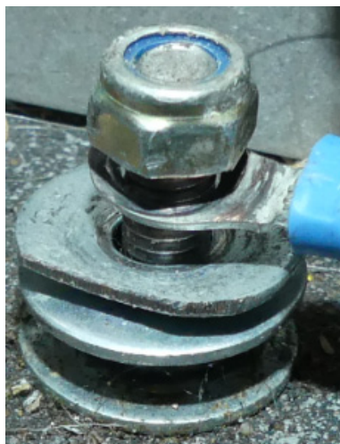
Illustration 7: The threaded bolt with the damaged washers and the cable shoe of the ground cable after the rectifier regulator had been removed
