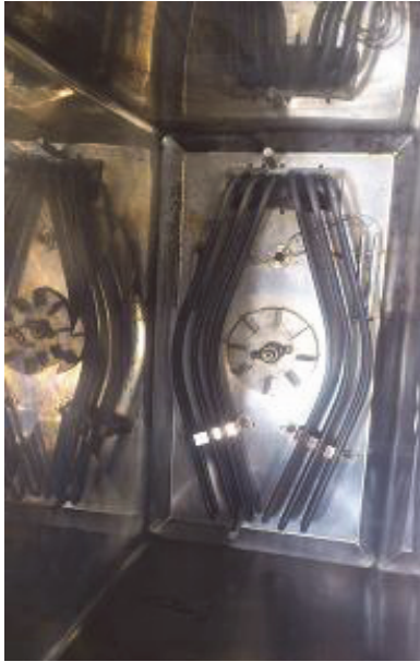
Figure 4: Oven with unprotected heating element
