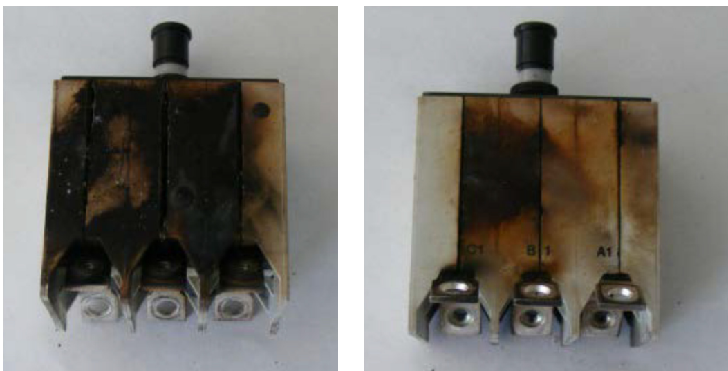
Figure 6: Front and rear of circuit breaker 3XN1 after the test (source: Airbus)
