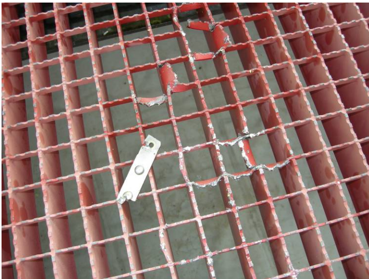
Figure 5: Torn out retaining clip and damage to grating
