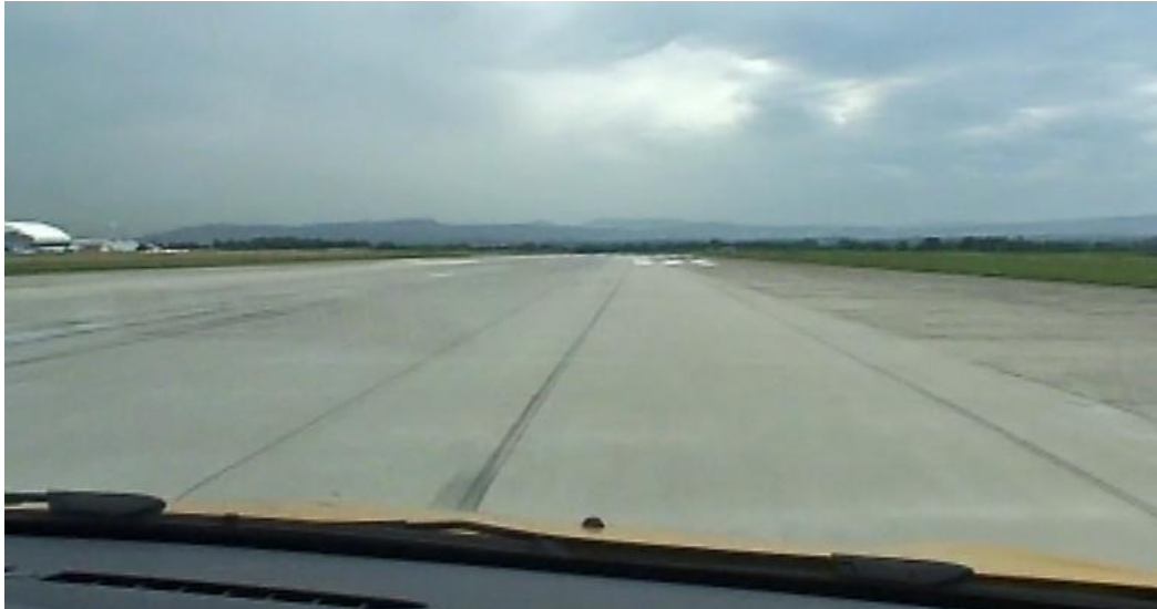
Fig. 4: Tyre marks on the runway
