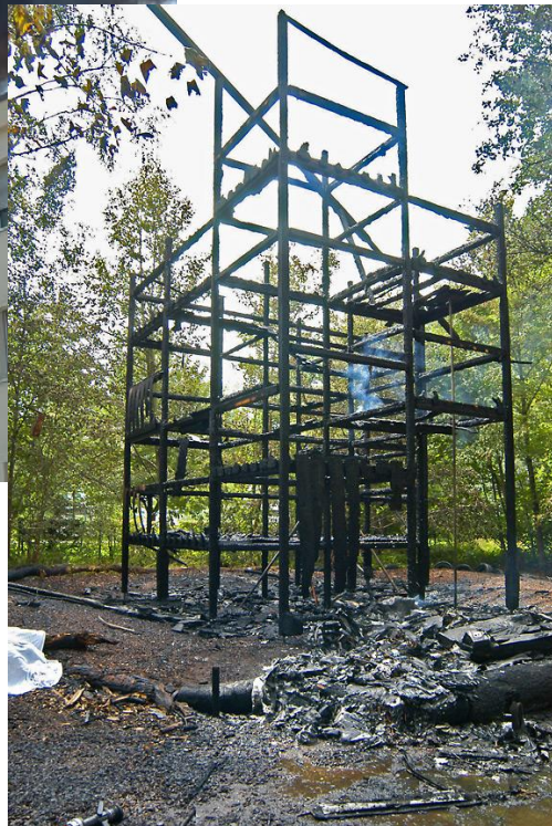
Fig. 8: Burnt-out climbing frame in the adjacent playground
