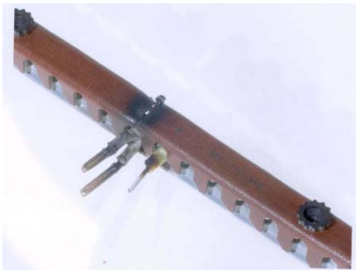
Fig. 2 Terminal Board with heat damage
