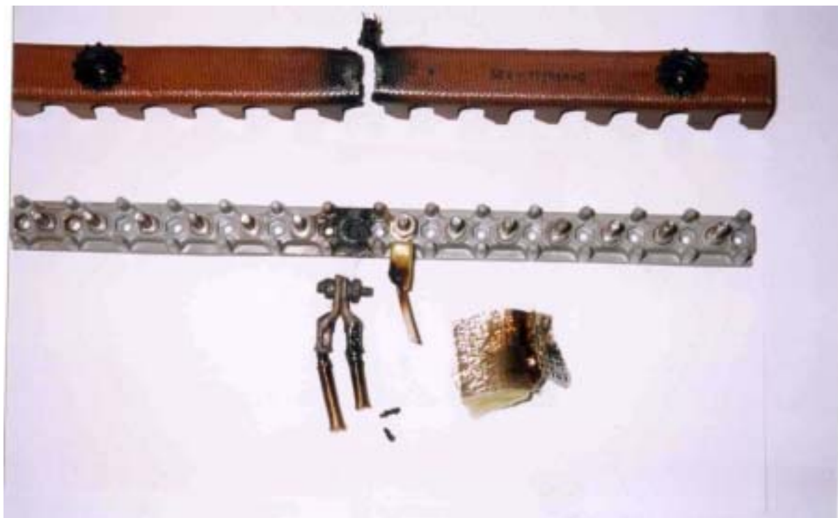
Fig. 3 Terminals with overheated connection
